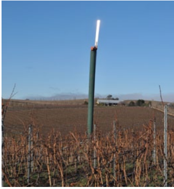
Plate 1: Fixed vertical fan system.
